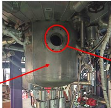
TOSQAN sump for under water test
